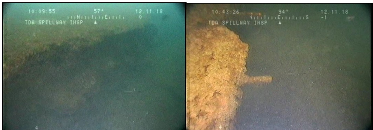
Figure 6 Images showing typical downstream apron end sill erosion along the entire apron downstream of Spillbays 1-8.
